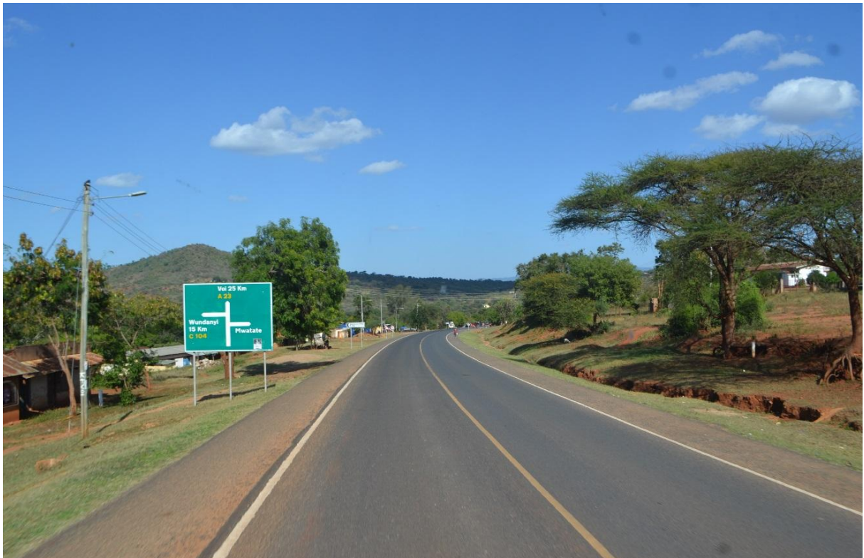
A section of the newly constructed Voi-Taveta road. On the right gullies are developing there is need to work on the drainage to protect the road from premature damage.
