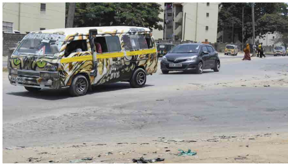
Figure 3: Deteriorated road surface at Makande Junction
