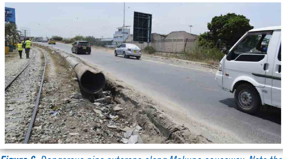
Figure 6: Dangerous pipe outcrops along Makupa causeway. Note the close proximity between the carriageway and railway line
