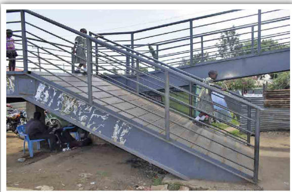
Figure 34: An abnormally steep ramp on the footbridge
