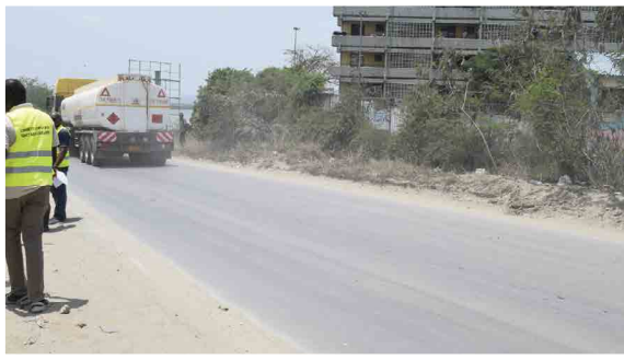
Figure 2: Missing road markings at Makupa Causeway
