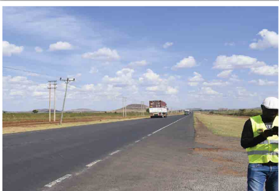
Figure 16: Long and straight stretch along Pipeline area. Faded road markings at the stretch also observed
