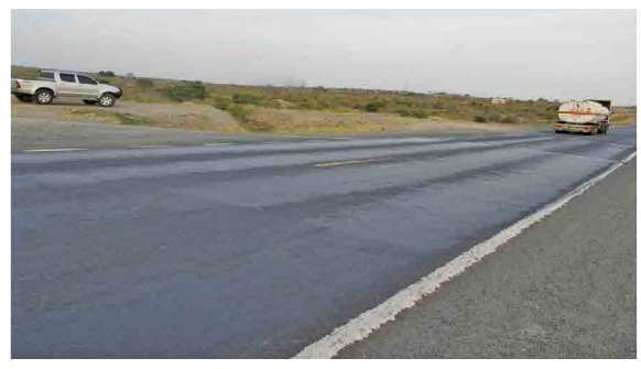
Figure 11: Bleeding road surface
