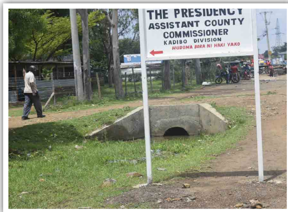
Figure 31: Silted/blocked access culvert
