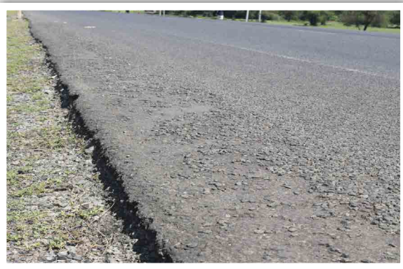
Figure 28: Hanging road shoulders
