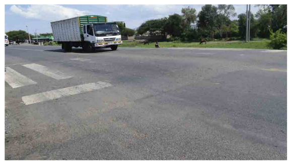
Figure 27: Faded road markings at a pedestrian crossing
