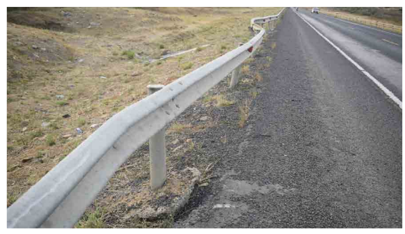
Figure 13: Damaged safety fences/guard rails
