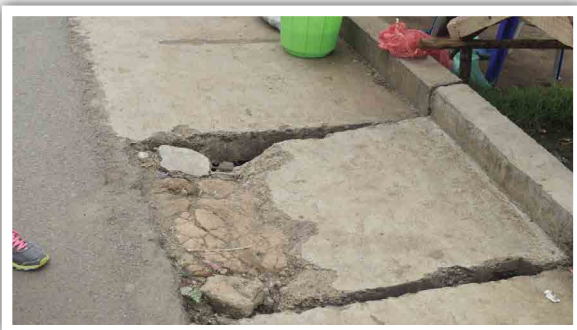
Figure 32: Damaged slab over a covered storm water drain
