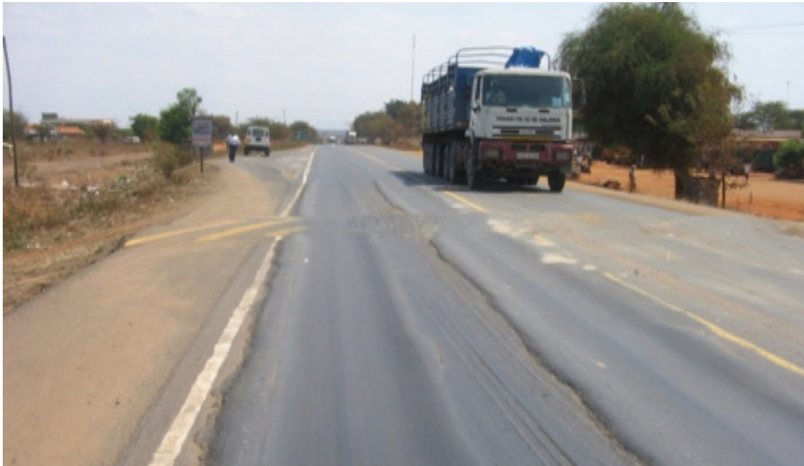
Figure 2: Overloading leads to increased damage to the road asset
