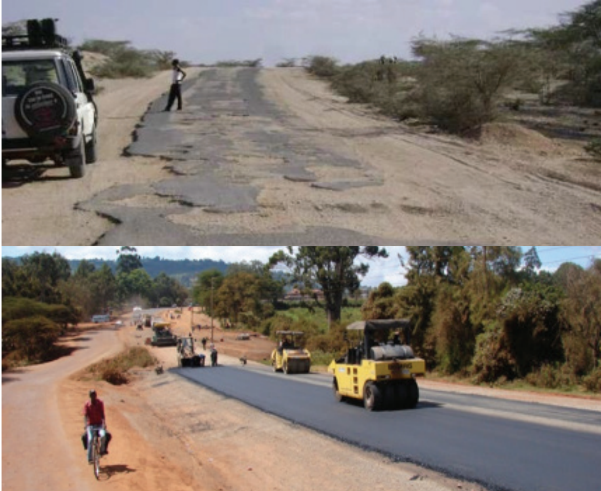
Figure 6: Costly and regular maintenance works
