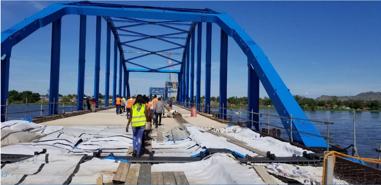
Juba new bridge still under construction. The new bridge will have a higher vehicle load limit than the old bridge.
