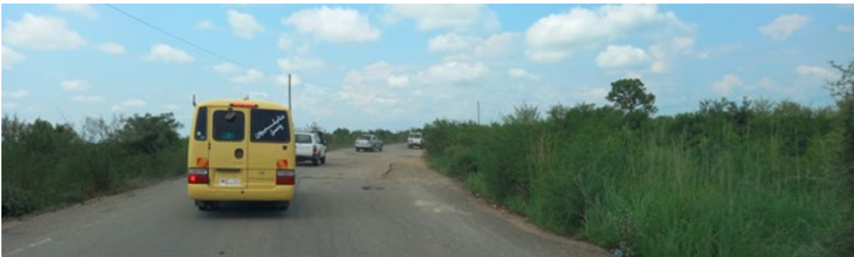
The Juba – Nimule Road less than 10 years after upgrade has suffered severe damages majorly due to overloaded trucks
