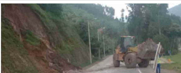
A grader clearing the road after a landslide along the Kigali-Rubavu road. The Survey Team also encountered several landslides along the Kayonza-Bujumbura road after Kayonza town towards Bujumbura. With heavy rains due to the topography of the area several landslides occur which affect flow of traffic along these transit sections.
